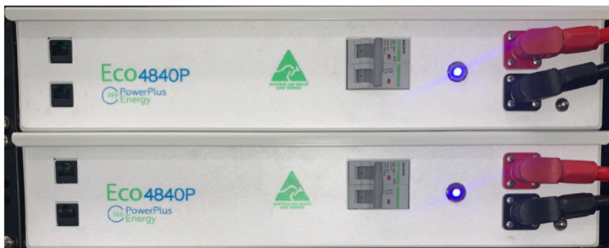
Battery Circuit Breaker ON
