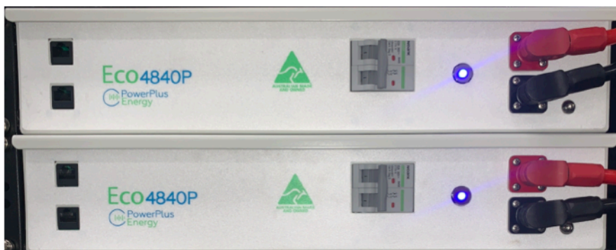
Battery Circuit Breaker ON
